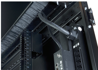
Series rack with 2 installed Eaton ePDUs
